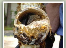
Grease clogged pipe
