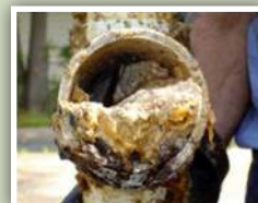
Grease clogged pipe
